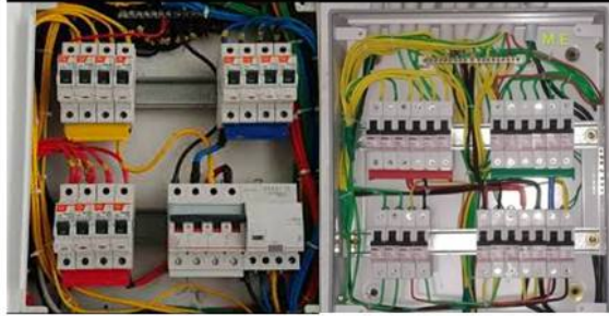
Figure 2.1.19: Electrical Control Panel
